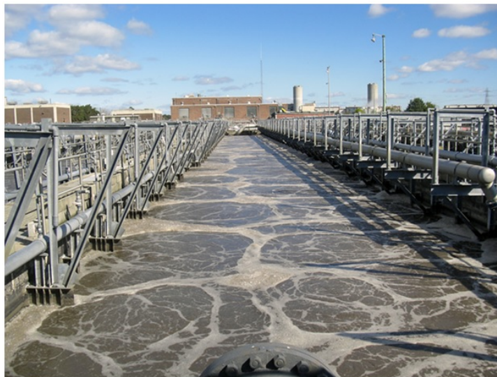
Activated Sludge Aeration Tank
